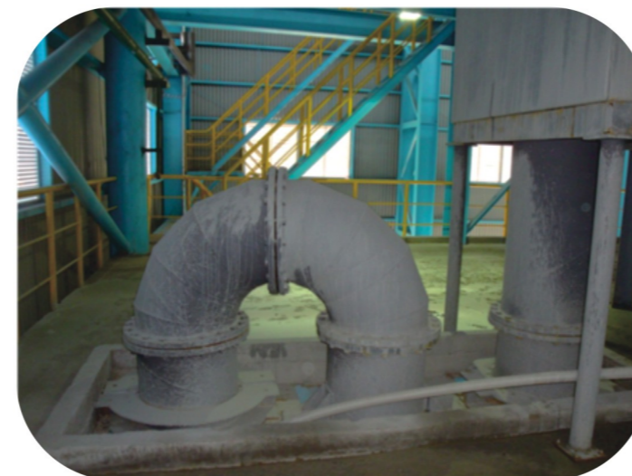
Rubber-lined pipe used on site
